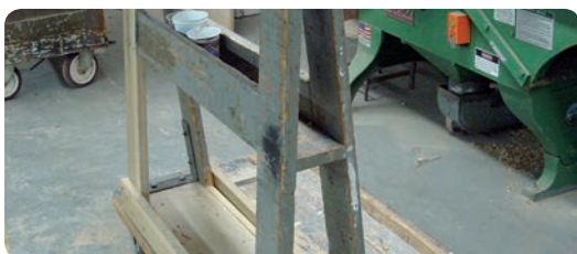
Wood - Splinters and rots
